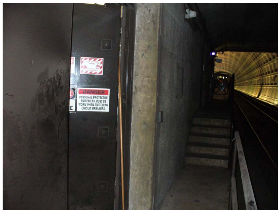
TIE BREAKER ACCESS
