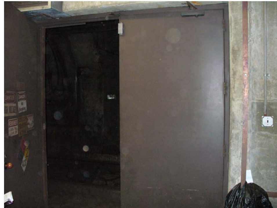
TIE BREAKER ACCESS
